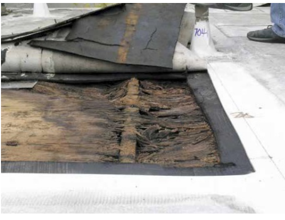
FIGURE 9. Image showing the damage caused by condensation build up on the wood deck. Image from Phil Dregger, vice president at Salas O'Brien Company.
